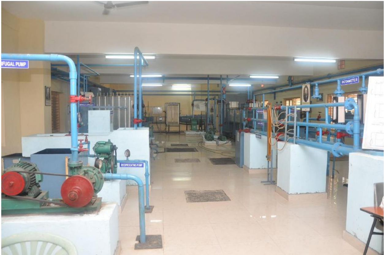
Fluid Mechanics and Hydraulic Machinery Laboratory
